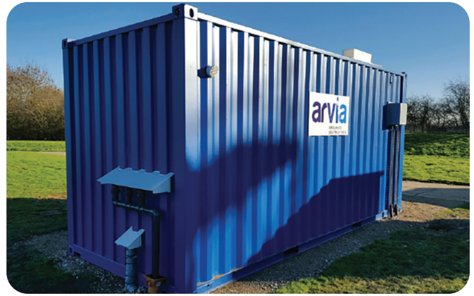
Containerised Nyex™ Treatment System on site at Anglian Water
